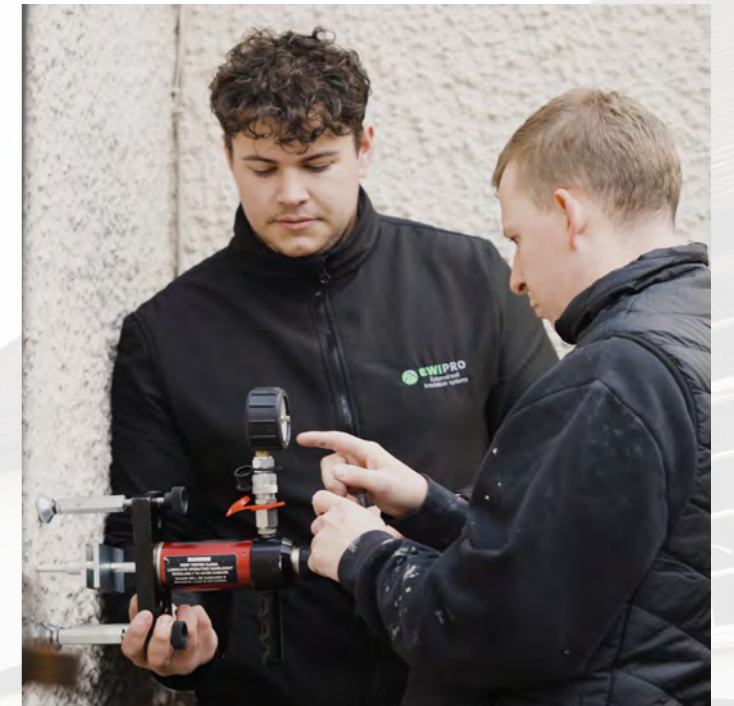
Pullout Testing - Josh from our BDM team supporting an installer with Pull Out Testing.
